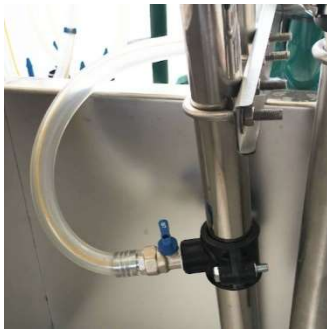
Valve inside wash bin
